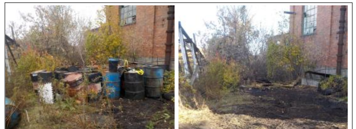
Before and after photos of one of the main drum storage areas. Photo credit: WWC Engineering
